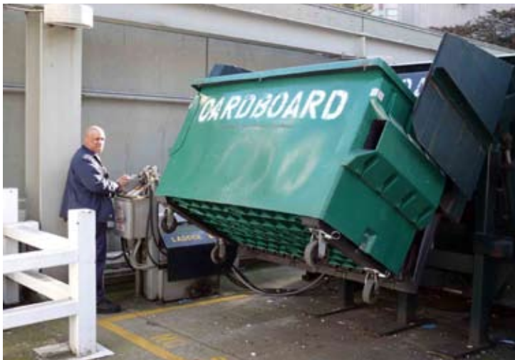
Large compactors are located at each of the Center’s two loading docks.
